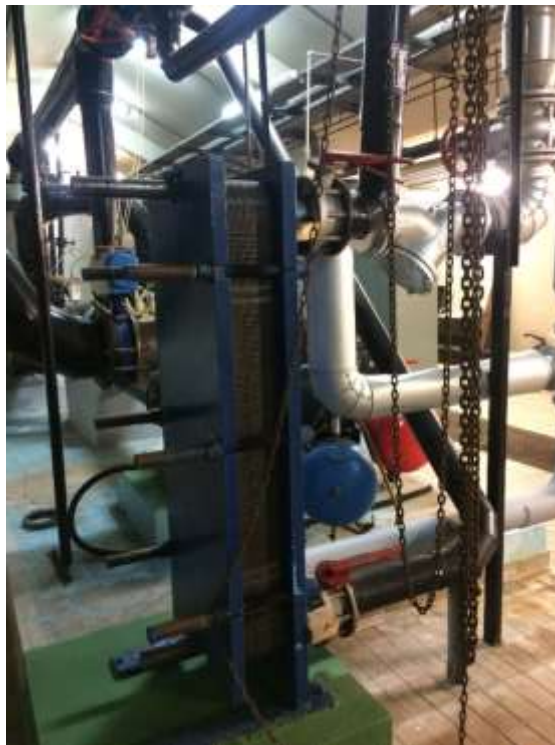
Heat exchanger at the heat center of Mladost cascade system, Croatia
